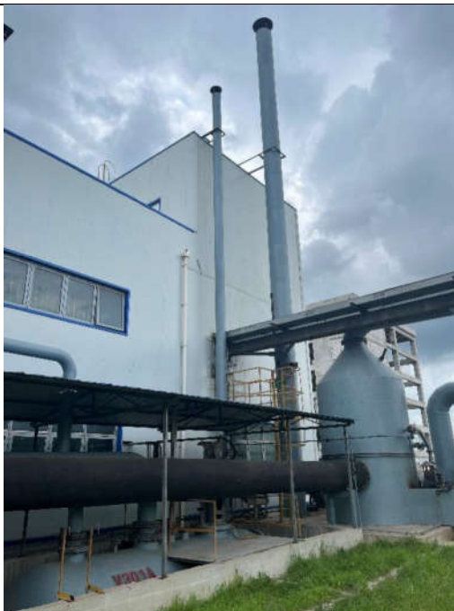
碱喷淋+活性炭吸附+DA007排气筒
